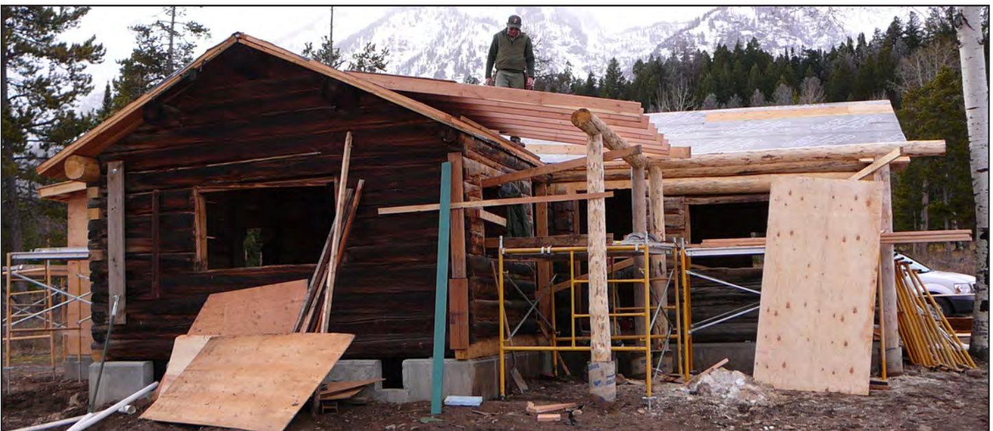
Above: 2011: new foundations, log replacement in-kind, and a new roof and porch.
