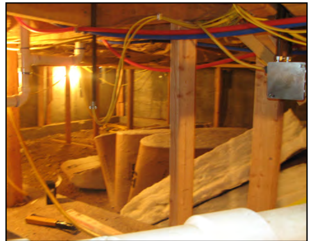
During the winter of 2012-spring of 2013, rotted floors were replaced, and new electrical, plumbing, heating and fire detectors were installed.
