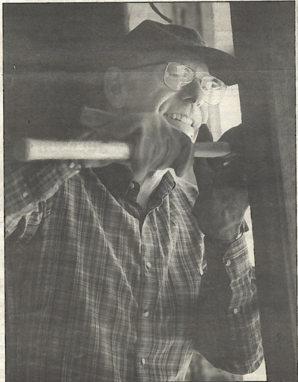
Helping with restoration efforts on the back porch, Howard Sloane pries at a rotten door jamb.
