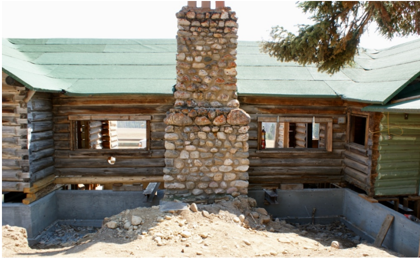
Back side of Main Cabin on I-Beams raised 3-4" while old foundation is removed and new concrete foundation built, 2012.
