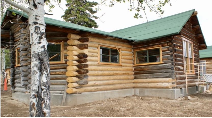
New logs replaced the sliding glass door taking exterior to back to 1950 Period of Significance.
