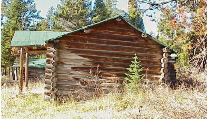
Cabin 1163's sinking, faulty foundation with dirt from spring runoff overtaking lower sill logs (R), circa 2002.
