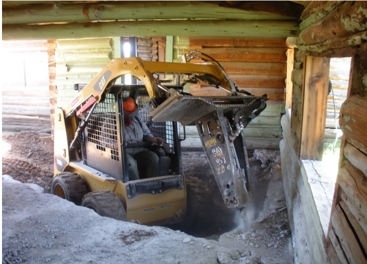
Removing 12" concrete inside the kitchen in preparation for a new foundation and crawlspace for modern utilities, 2012.
