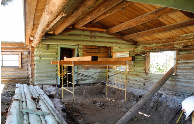
Old kitchen roof supported as original rotten logs on three sides were removed, 2011.
