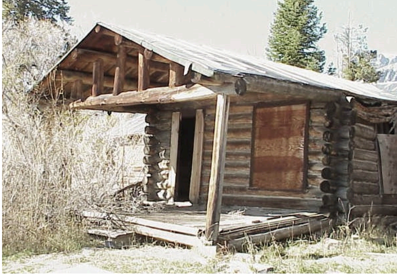
Hammond Cabin pre-rehabilitation with crumbling foundation, deteriorated exterior log walls, leaking roof, rotted windows and fallen floors internally, 2006.
