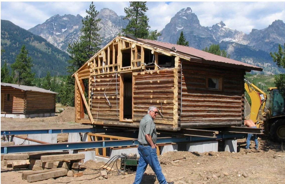
Once the buildings were relocated to Beaver Creek (park residences), they were placed on new foundations. Photo courtesy of WCHP 2005.
