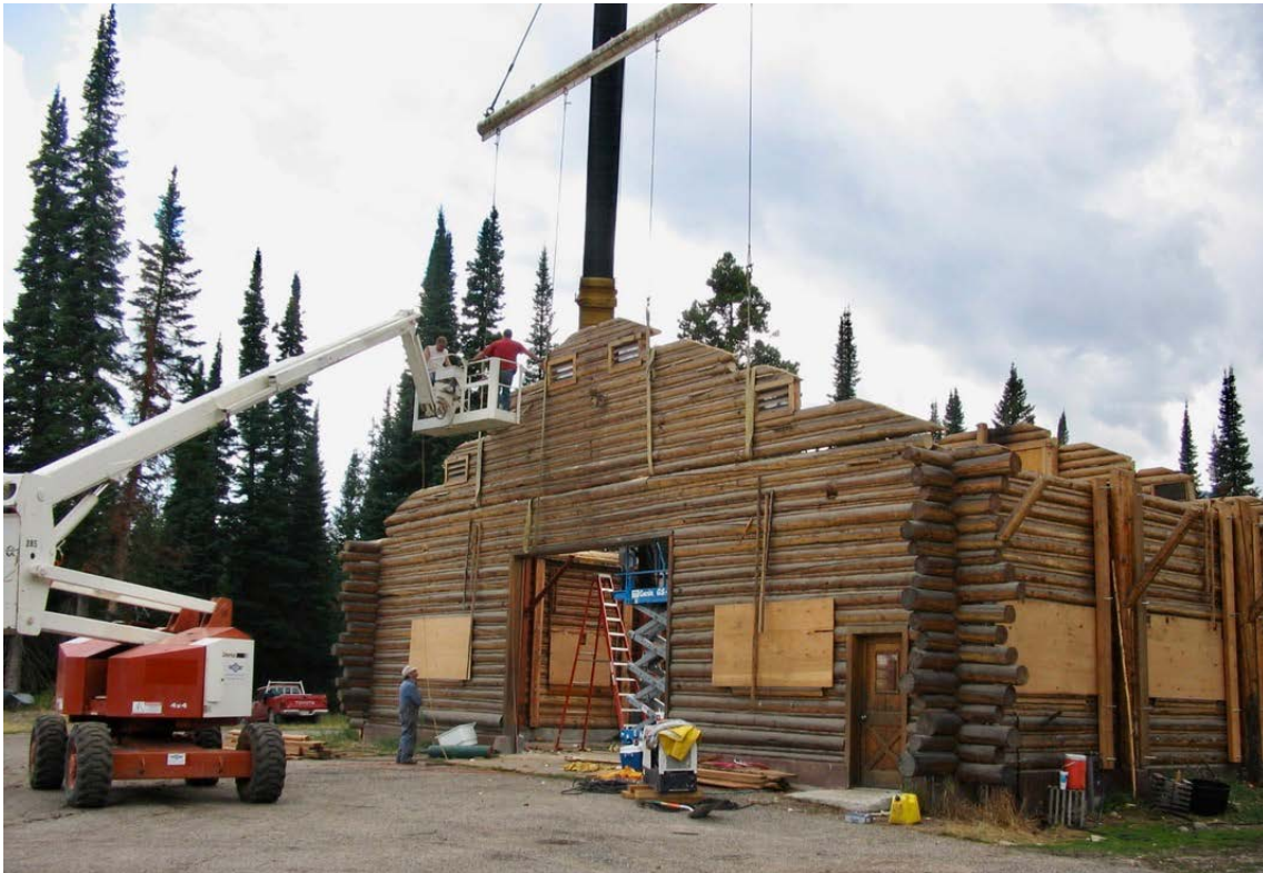
Preparing to lift the gable section of the roof and place it on a truck for transport. Photo courtesy of WCHP.
