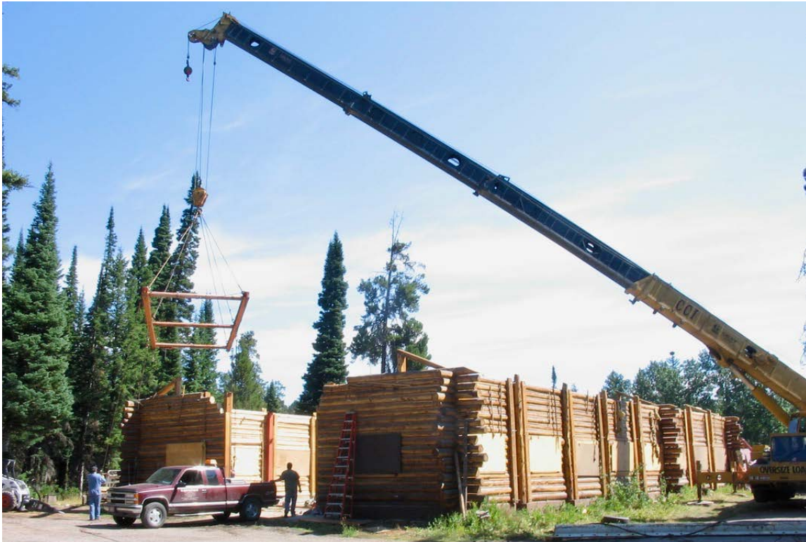
Roof and its steel structure removed; two ends and two sides remain to be taken apart and moved to Moose. Photo courtesy of WCHP, 2005.
