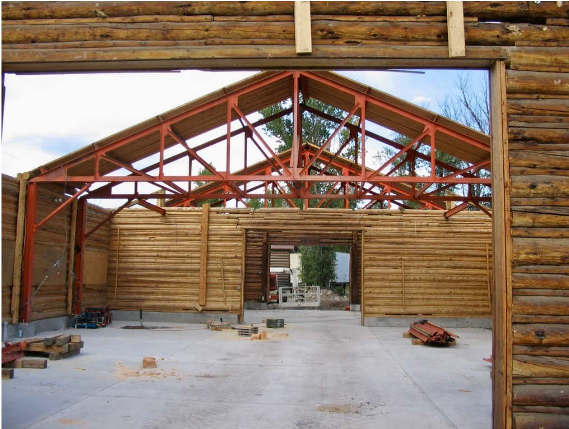
Interior wall now in place separating shop space from WCHP offices. Photo courtesy of WCHP, 2005.
