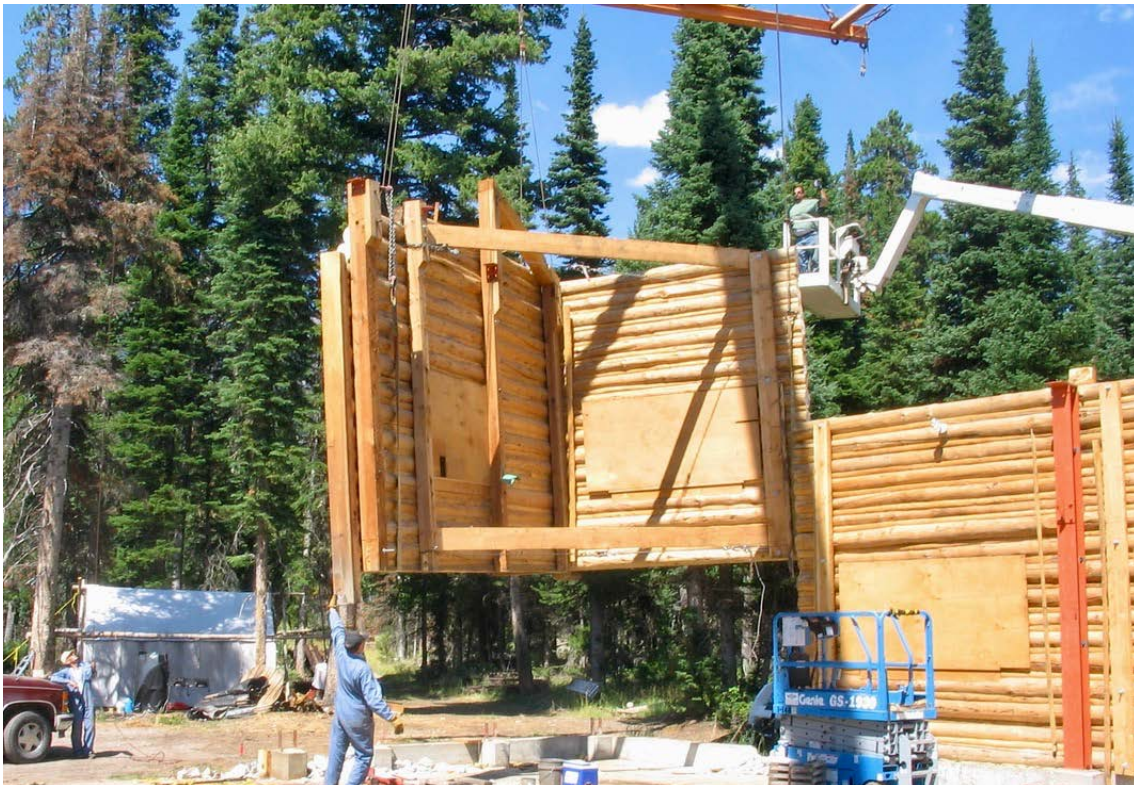
Lifting a corner of the Shop for placement on a truck. Photo courtesy of WCHP, 2005.
