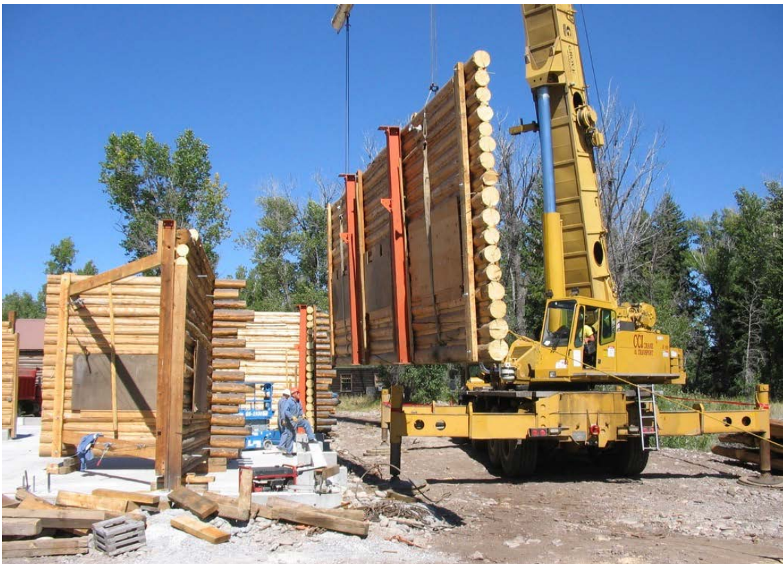
Lifting a wall section attached to its steel structure for transport to Moose. Photo courtesy of WCHP, 2005.
