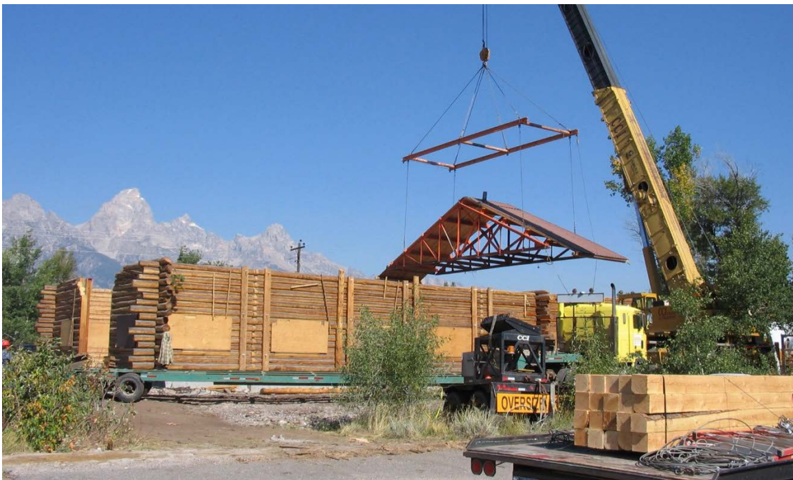
Once in Moose, the walls have been erected/secured, the crane lifts the first section of roof for placement. Photo courtesy of WCHP, 2005.
