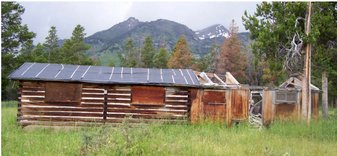
Girls' Cabin at White Grass with Visqueen cover to protect roof. Photo courtesy of WCHP 2002.
