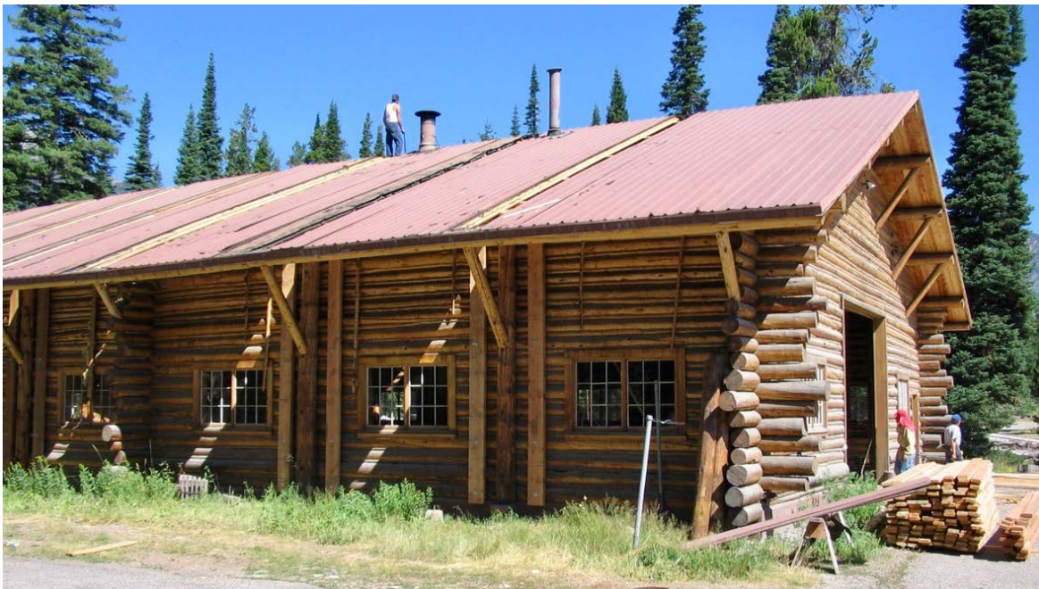
Dismantling the JY Shop in preparation for move to Moose. Photo courtesy of WCHP, 2005.
