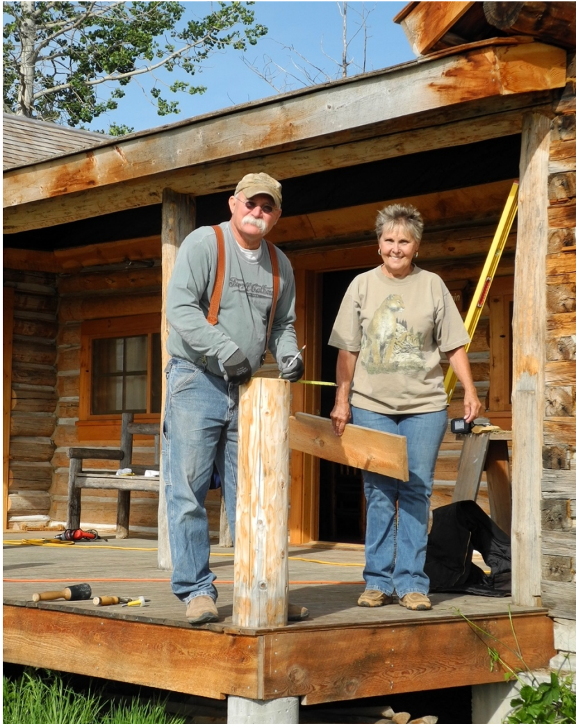
Carpenters William 'Dub' Lloyd (Wrangler, 1983) and Marilyn Smith volunteer their services at White Grass during summers 2017-2019. In photo above, they are constructing a log hand railing for the rehabilitated Main Cabin front entrance.
