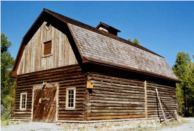
Rebuilt Barn using as much original material as possible including hand forged door hinges. Photo courtesy of Carole Hofley.
