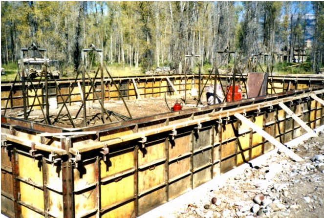
Building a concrete foundation according to local code. Photo courtesy of Carole Hofley.
