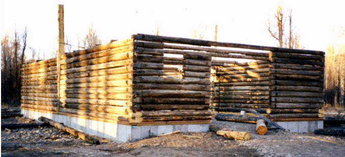
Bottom Logs reassembled. Photo courtesy of Carole Hofley.
