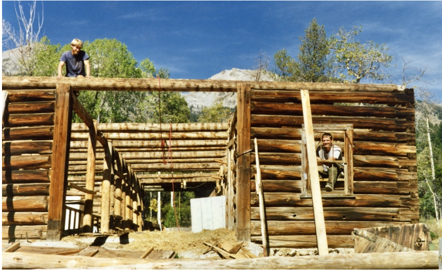
Reconstructed roof removed exposing the original log structure dating back the 1913-1919. Photo courtesy of Cavicchioni & Gerster.
