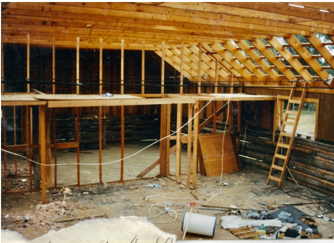
Upper portion of the barn above the horse stalls built, not part of the original structure. Photo courtesy of Cavicchioni & Gerster.
