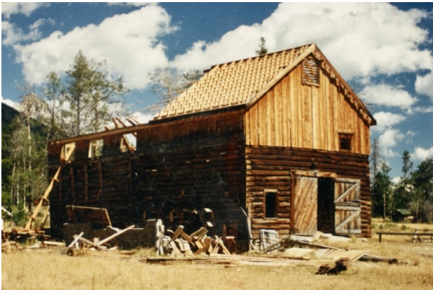
Barn with side shed dismantled and roof coming off. Photo courtesy of Cavicchioni & Gerster.
