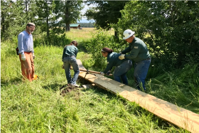
Foot Bridge across marsh area for trail access to White Grass. Built by Groundwork USA Volunteers, 2018. Photo courtesy of R. Butterbaugh.
