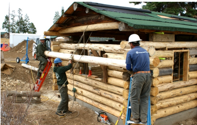
Roger Butterbaugh (R) helping others install a new log on the Main Cabin Kitchen, 2012. Photo courtesy of Craig Struble.
