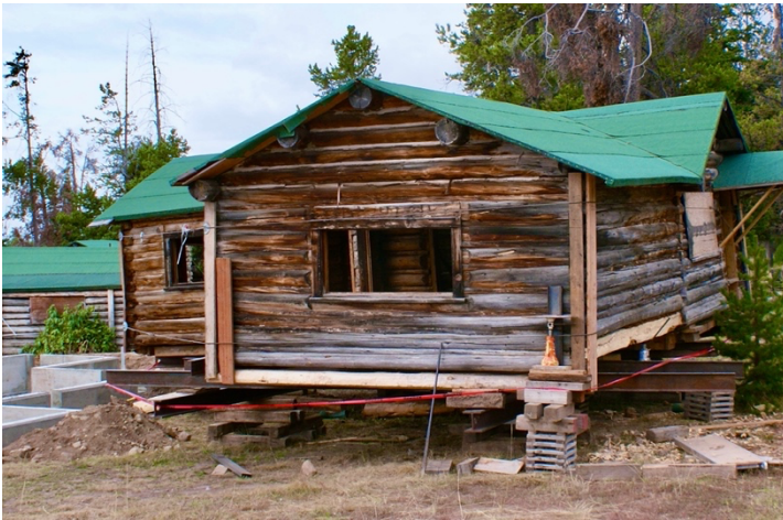
Cabin 1158 elevated and moved to create new foundation; lower sill logs replaced. Photo Courtesy of R. Butterbaugh, 2010.
