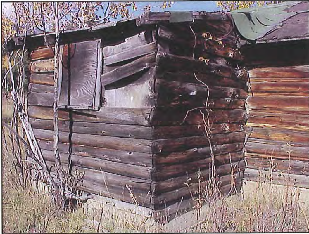
Figure 58. Detail of bathroom addition on the south side of HS-1160, Cabin 8. Source: A&E Architects, 2004.
