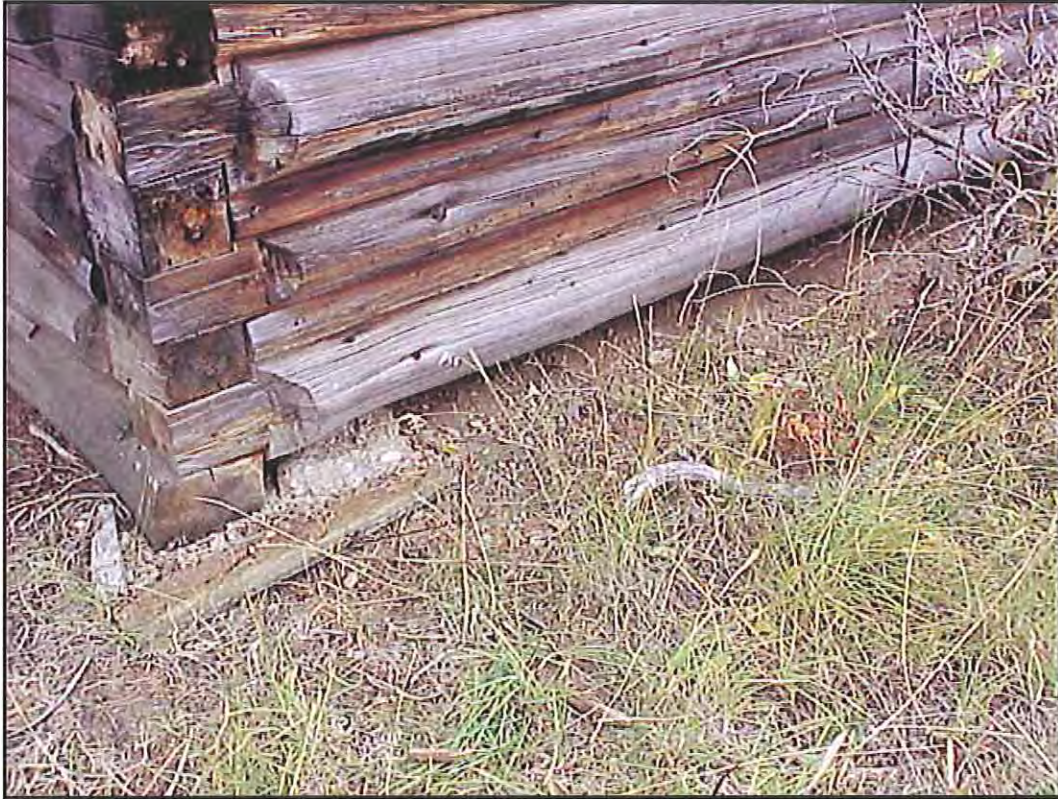
Figure 28. Detail of deteriorated foundation pier, HS-1155, Cabin 15. Source: A&E Architects, 2004.
