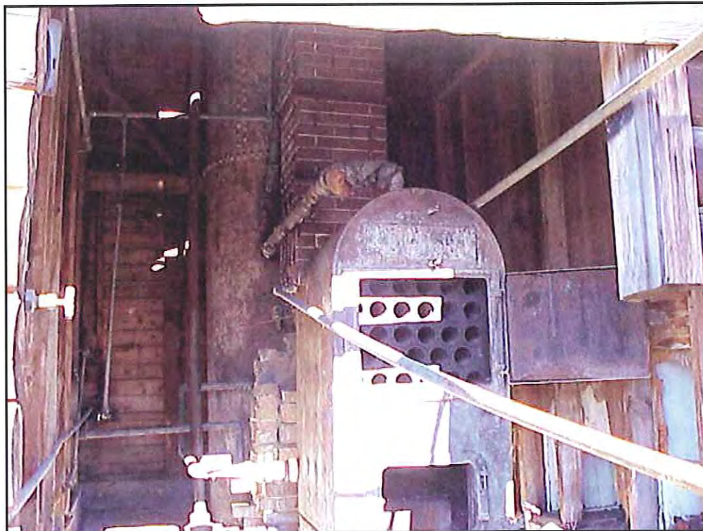
Figure 69. Interior of the east room of HS-1162, the Bathhouse. Source: A&E Architects, 2004.
