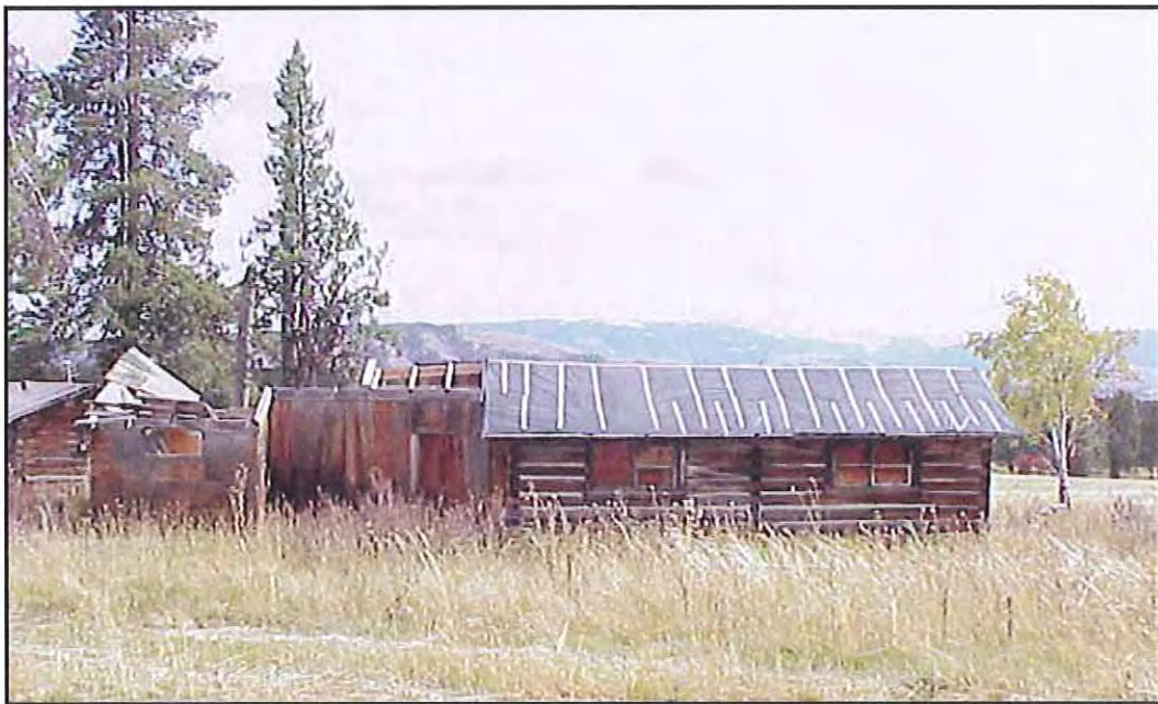
Figure 22. Looking east to the west wall of HS-1154, Girls' Cabin. Source: A&E Architects, 2004.
