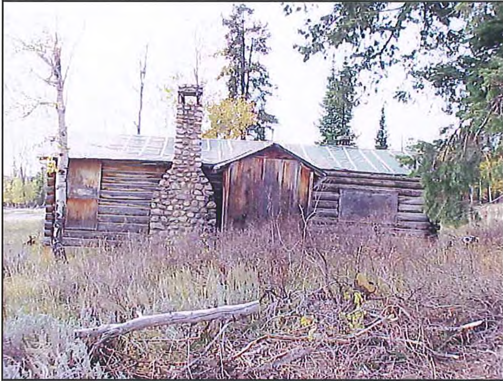
Figure 32. North wall of HS-1156, Hammond Cabin; the frame addition in the approximate middle of the wall contains a bathroom. Source: A&E Architects, 2004.
