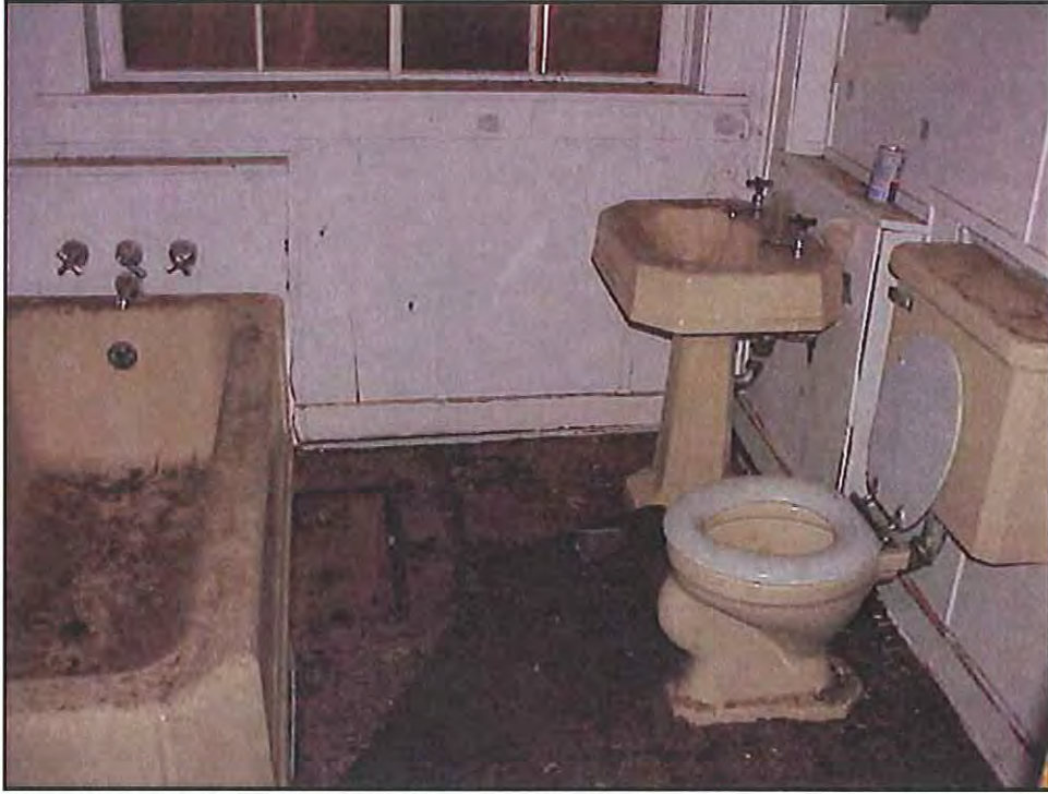
Figure 36. Detail of the interior of one of the bathroom additions, HS-1156, Hammond Cabin. Source: A&E Architects, 2004.
