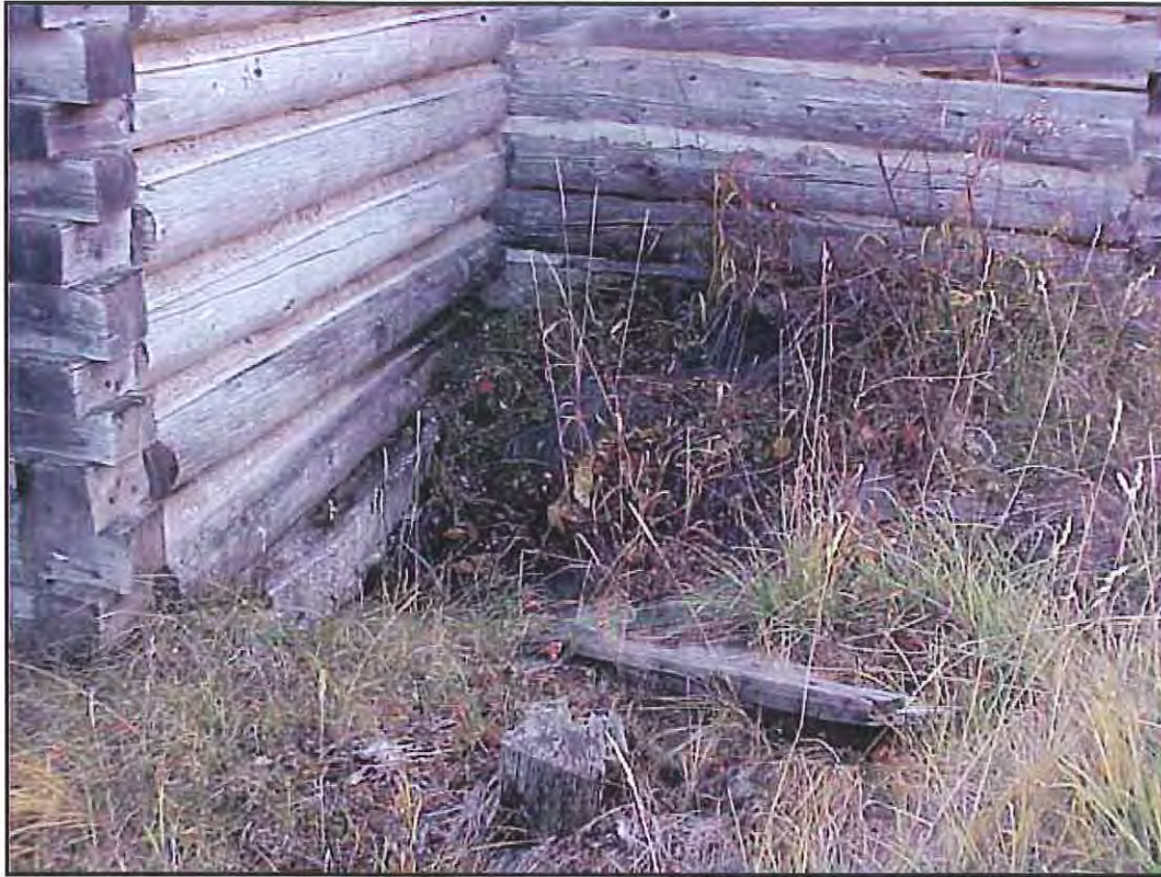
Figure 63. Detail of the junction of the addition (left) and the main volume (right), showing differences in daubing. Source: A&E Architects, 2004.
